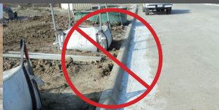
Illegal discharge to storm sewer!
