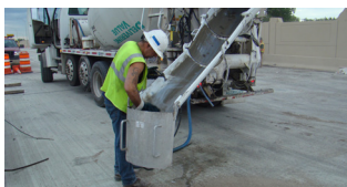
Chute washout system.
