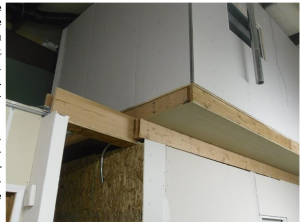
What's really holding this mezzanine up? How do you get up there? What if the fire is inside the mezzanine room?
